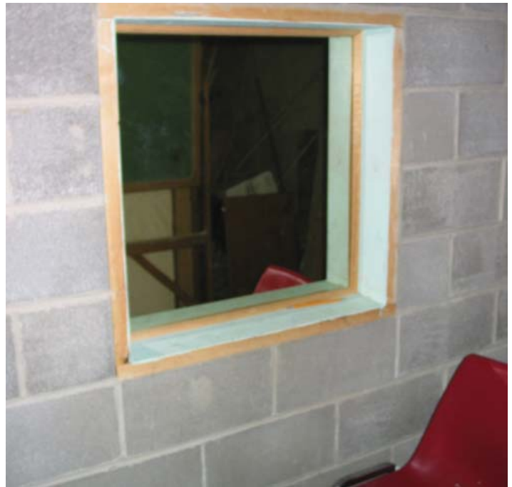
A seclusion room in a basement of a school in southwest Ohio.
